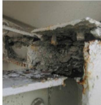
Topical bad rust
